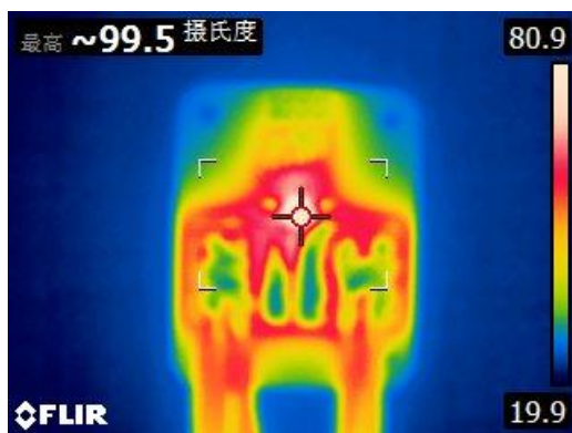
Package Thermography (Input Current 40A)
